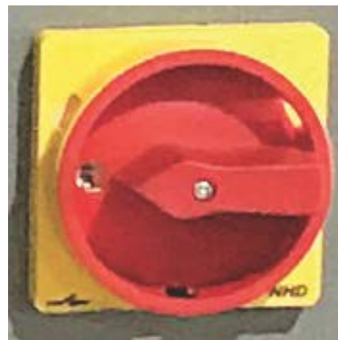
Figure 9-2: Main Power Switch
