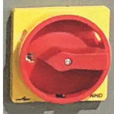
Figure 9-2: Main Power Switch
